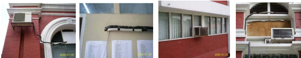
Figure 7: Poor planning and installation of outdoor air conditioning unit which affected the buildings' façade; (i) exposed of outdoor unit, (ii) poorly enclosed of existing window
