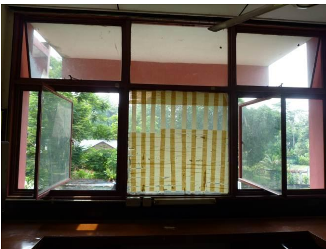
Figure 9 Two types of windows namely, centre pivot and awning which are glass tinted with biggest window area at K3
