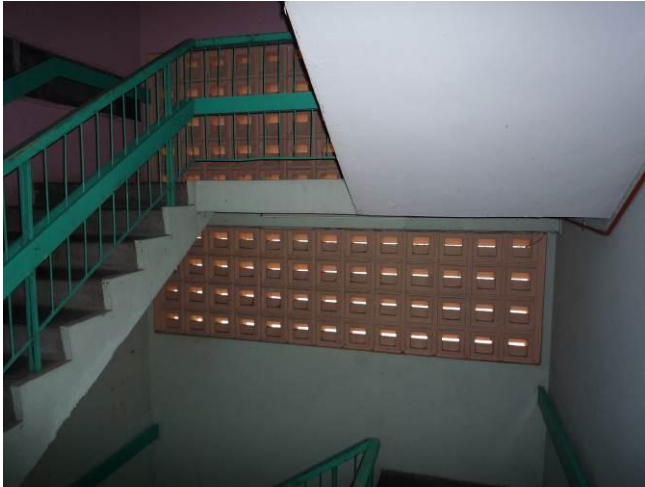
Figure 6 Fixed opening devices in larger scale at the staircase area of K1.
